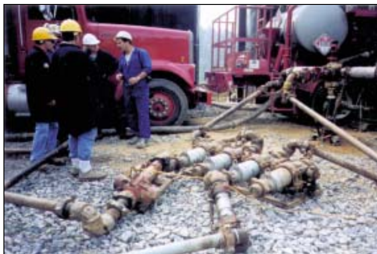
Figure ES-6. The fracturing fluids, additives, and proppant are pumped from the storage tanks to a manifold system placed on the wellhead where they are mixed just prior to injection.
