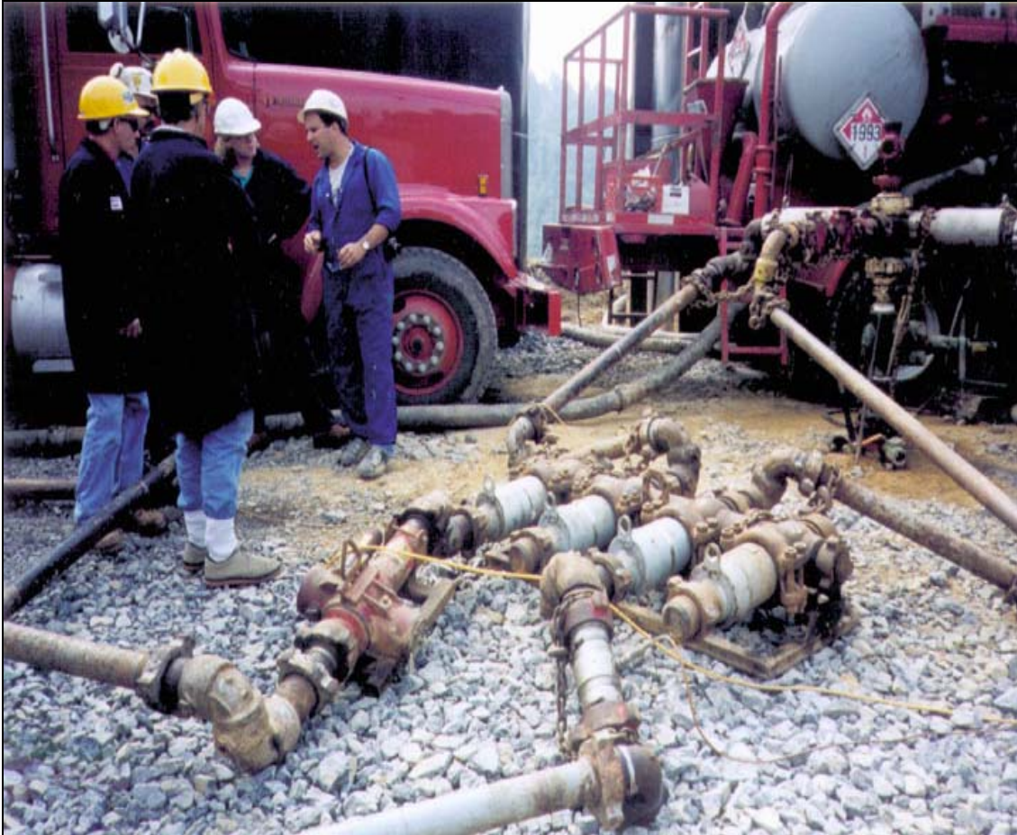
Figure 4-7. The fracturing fluids, additives, and proppant are pumped to the wellhead and mixed just prior to injection. The flow rate of each injected component is monitored carefully from an on-site control center.
